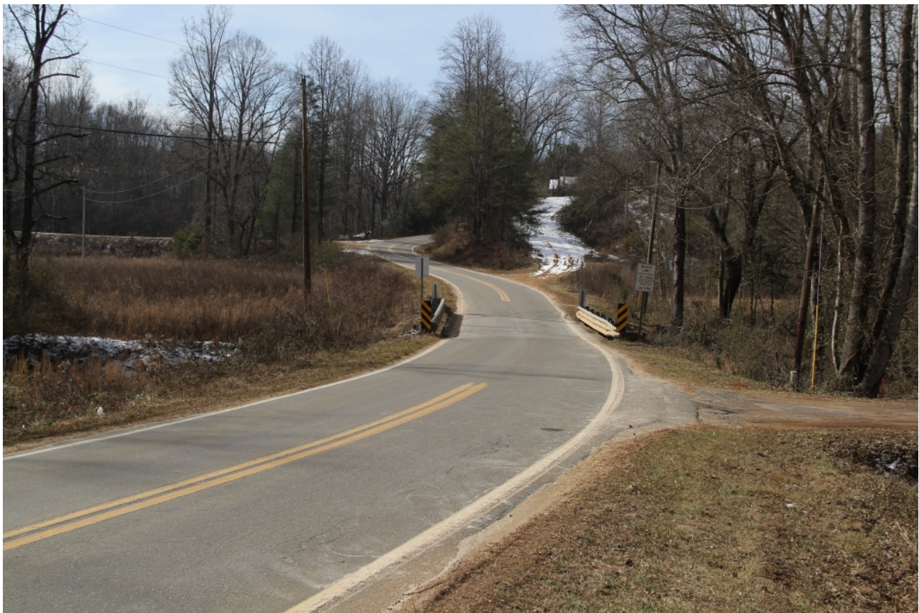
Bridge No. 34 on SR 1907 (Rhoney Road) over Rock Creek, view to southwest
